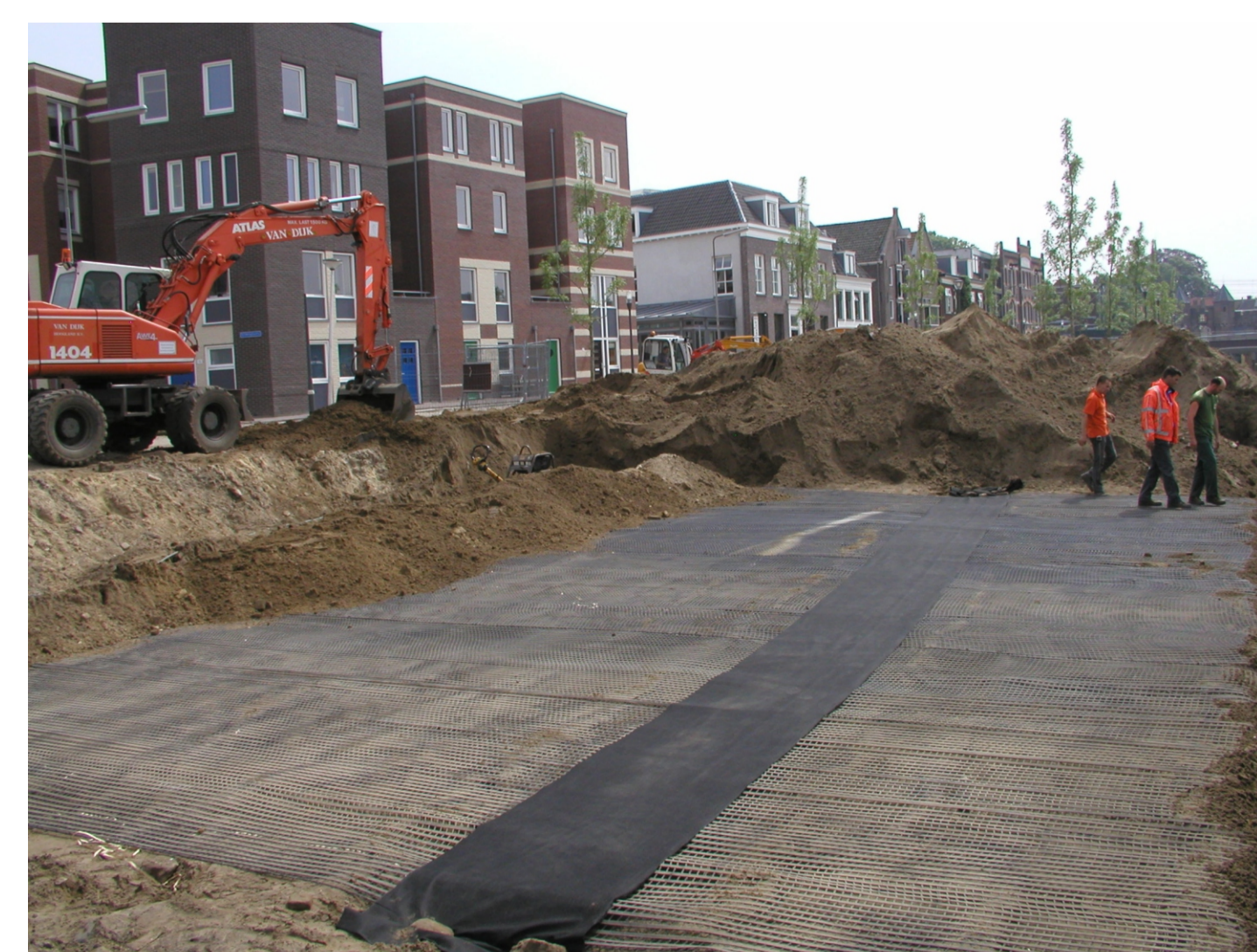
placing a non-woven over the trench to retain the sand on the geogrid
