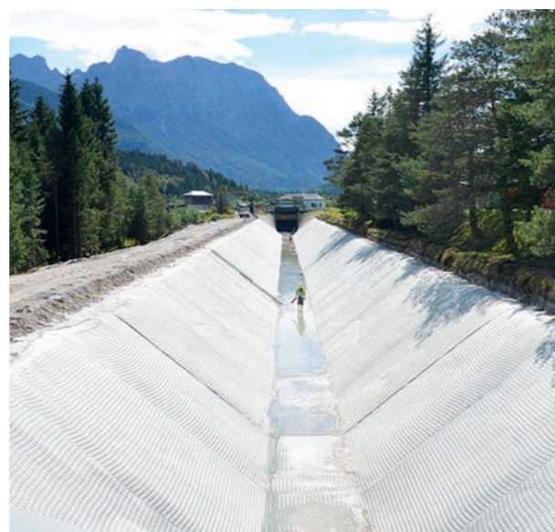
Canal refurbishment Germany, 2015, lining of Isar link canal using Incomat Standard geosynthetic concrete mattress.
