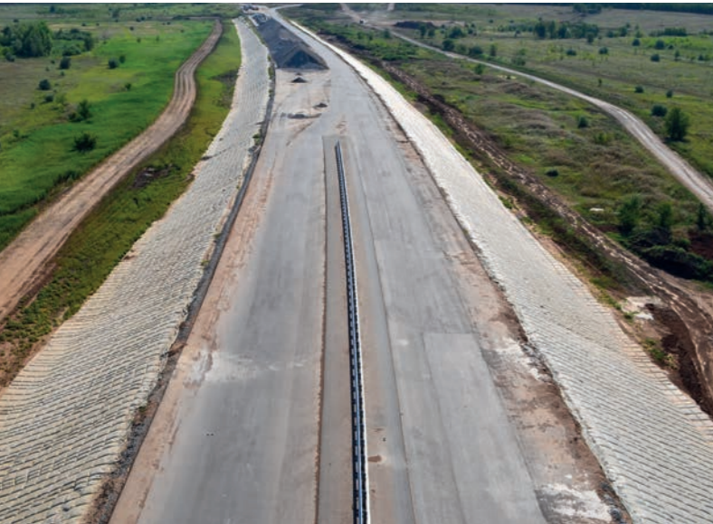
Embankment construction Russia, 2011 – 2014, protection of side faces of highway embankment slopes by Kirovsky bridge in Volga and Samara river floodplains using Incomat Flex.
