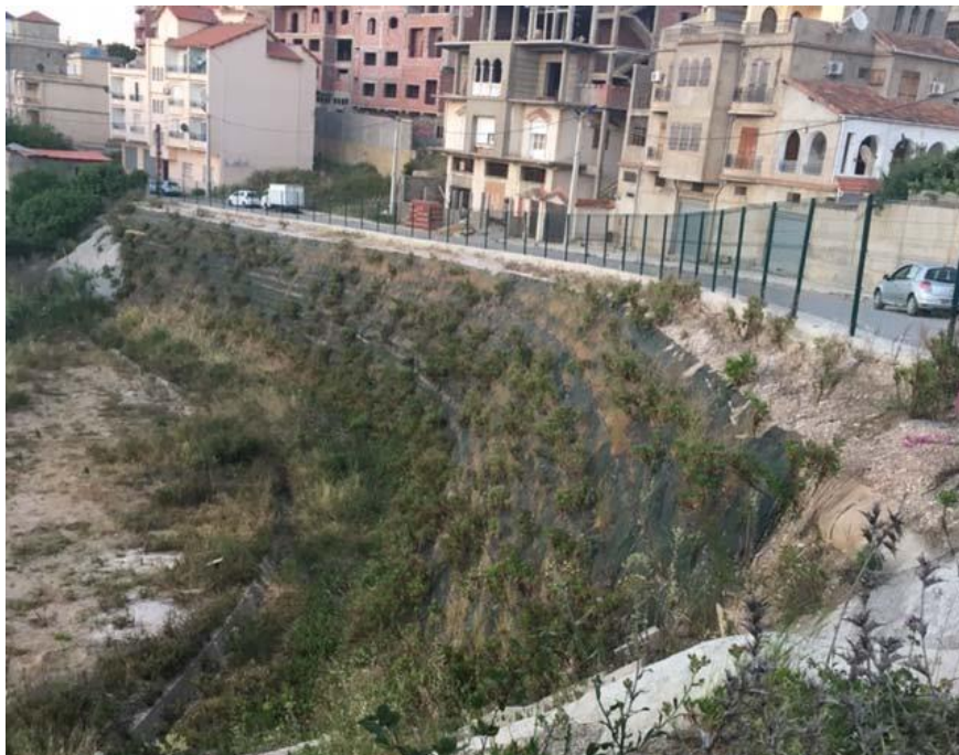
Figure 18. View of the GRS 3 years of the construction. Natural greening of the facing and no cracks on the street uphill
