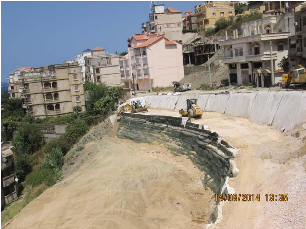
Figure 17. Building of the Geosynthetic-Reinforced Soil, layer by layer, filled by compacted material
