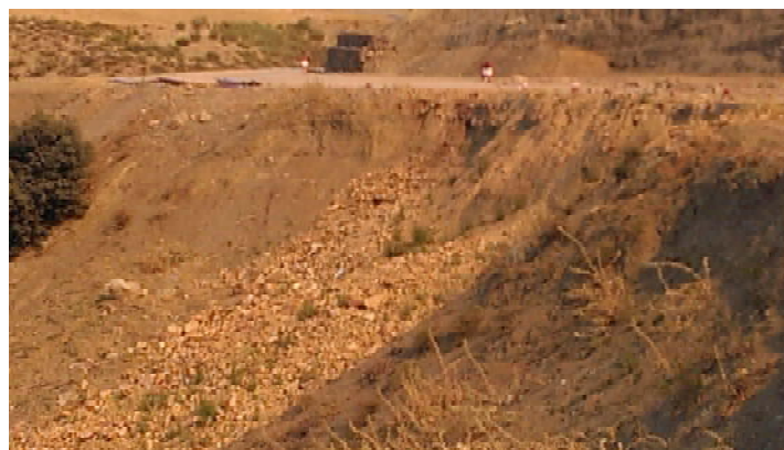
Figure 5. View of the road and the sliding before rehabilitation
